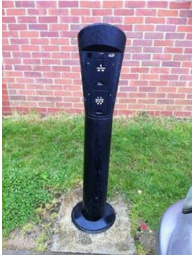
Example of an electric vehicle recharging point.
